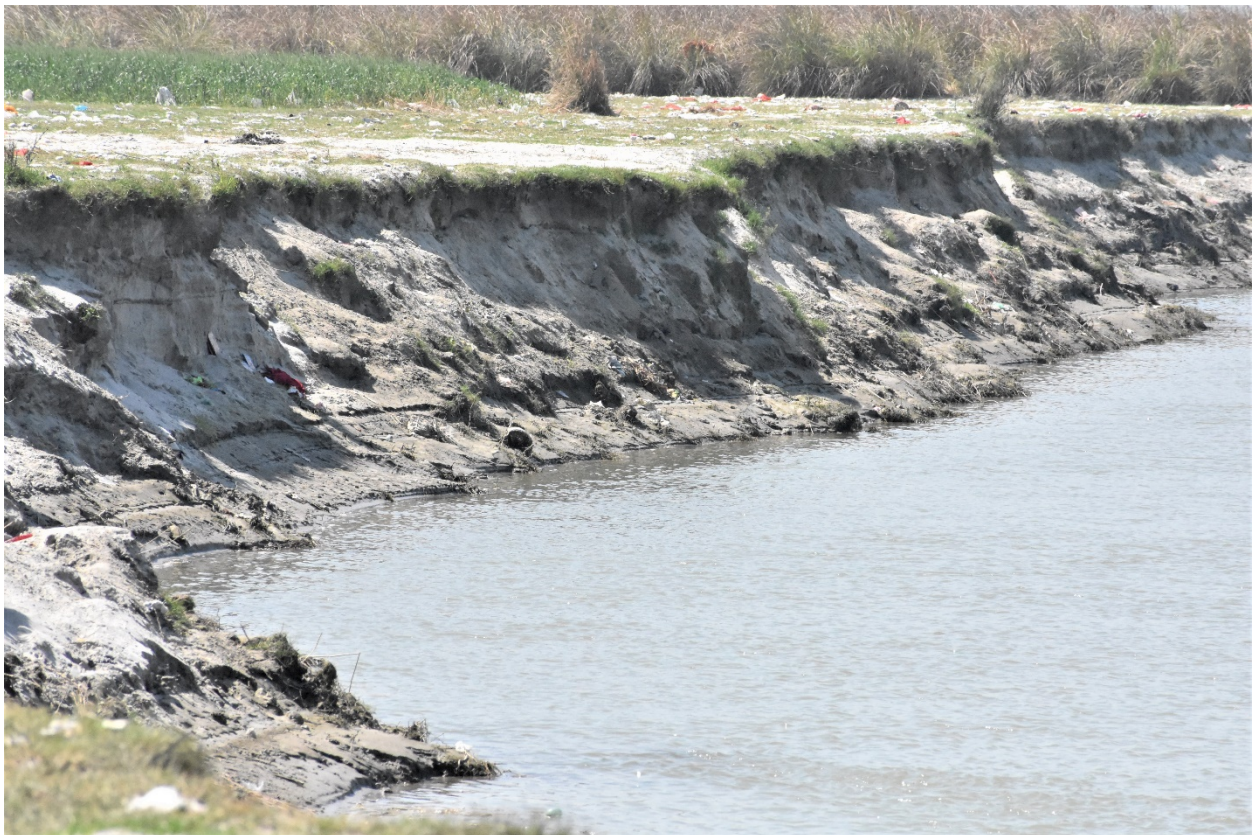
Image 30 : Ganga River Bank Erosion As Observed Near Lahara Ghat In Kasganj Distt.
